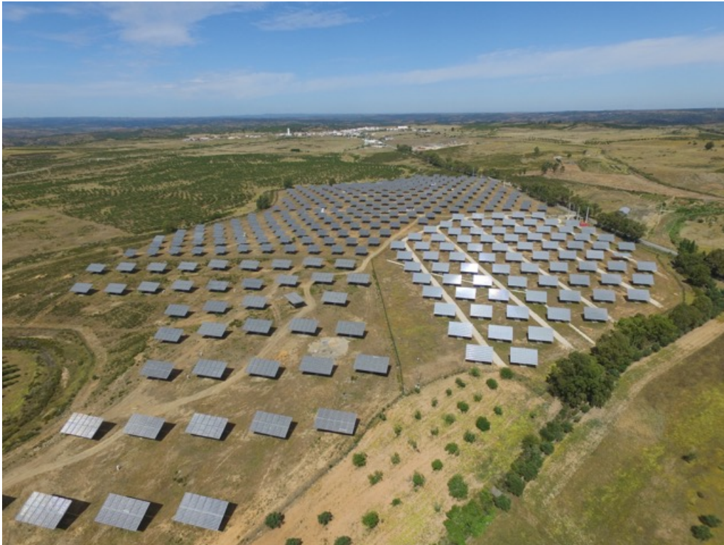
Figure 2-4. Picture of the SDP from air with the trackers visible (Enercoutim, 2016a).
